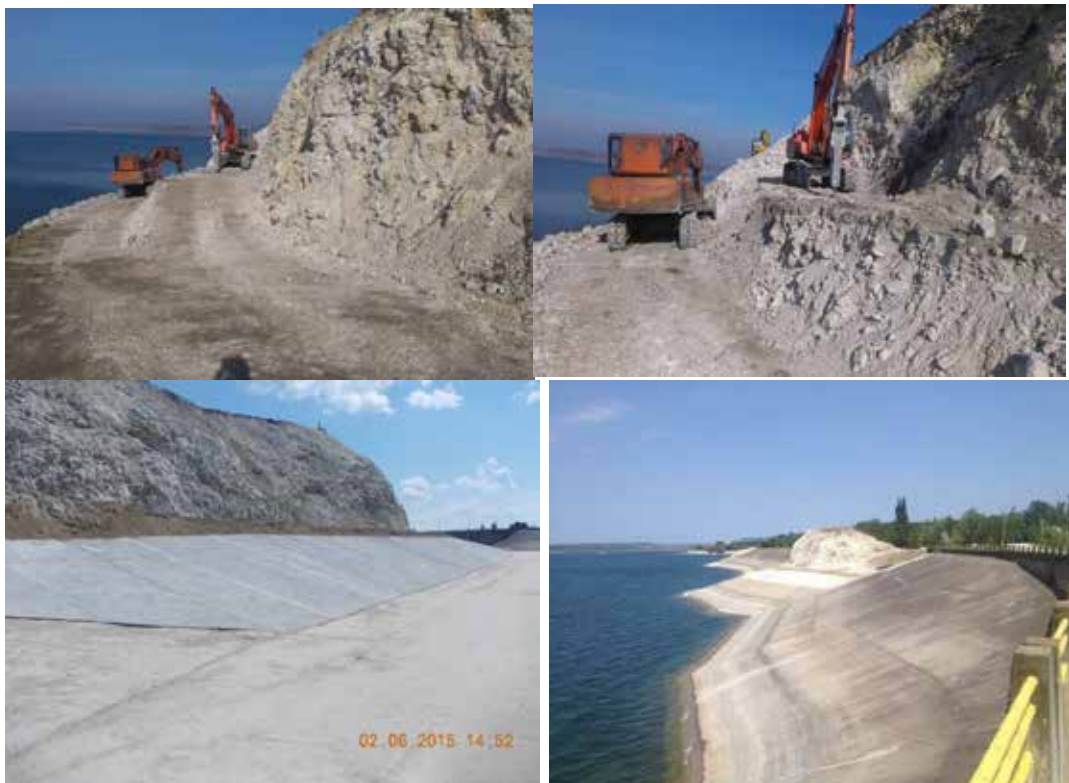
Reducing the slope and bank consolidation of two sectors of the reefs
