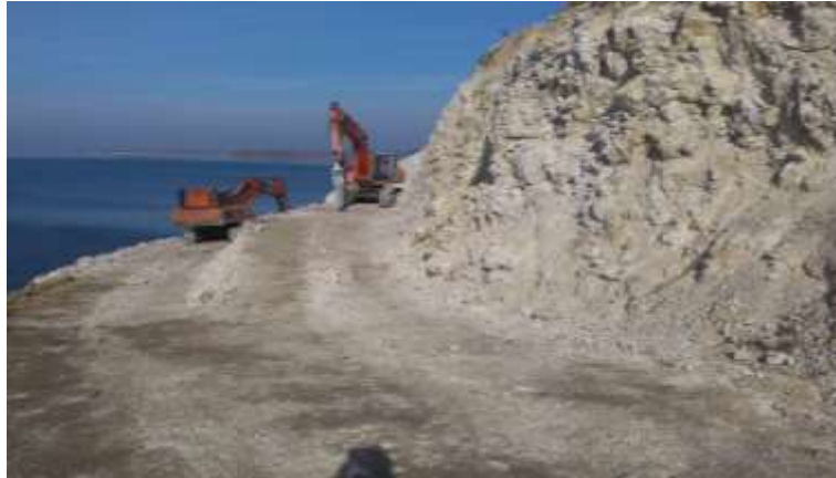
Figure 1. Reducing the slope and bank consolidation of two sectors of the reefs
